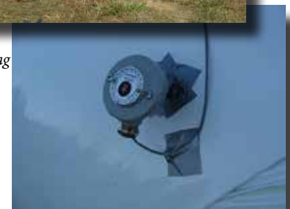
Right: Sensors on silo bags measure ambient conditions, temperature, airflow distribution, and CO 2
